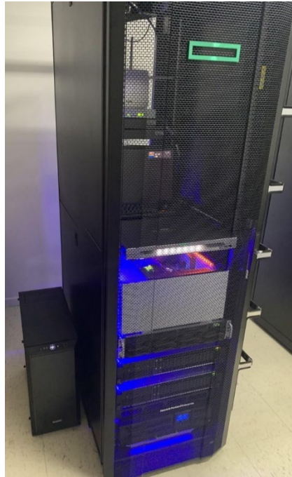
Figure 3. Hardware placement inside premise
