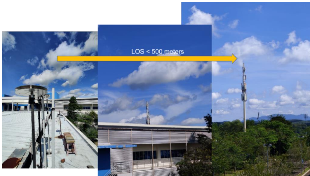
Figure 15. The telecommunication tower hosted U Mobile 4G equipment located less than 1 km from the lightning sensors
