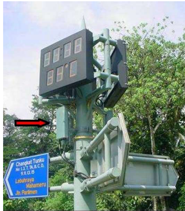
Figure 10. Panel antenna on a signage pole with clock
