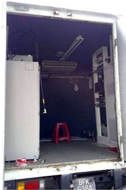
Figure 18. Interior of mobile BTS
