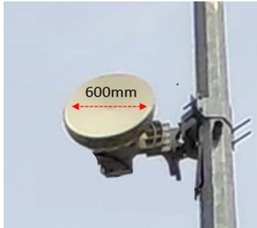
Type A1 - microwave dish mounted at new retrofit or existing structure
