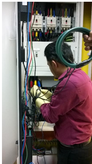
Figure 7.1 Data Logger installed at DB
