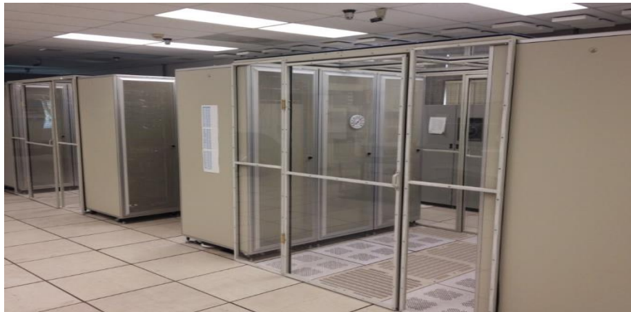
Figure 10.2 “Cold Aisle” configuration for Under Floor Air Delivery (UFAD) using fixed plastic sheets
