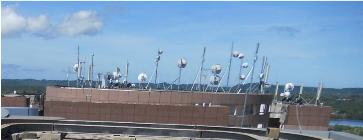
Figure 9.3 Base Transceiver Station on building
