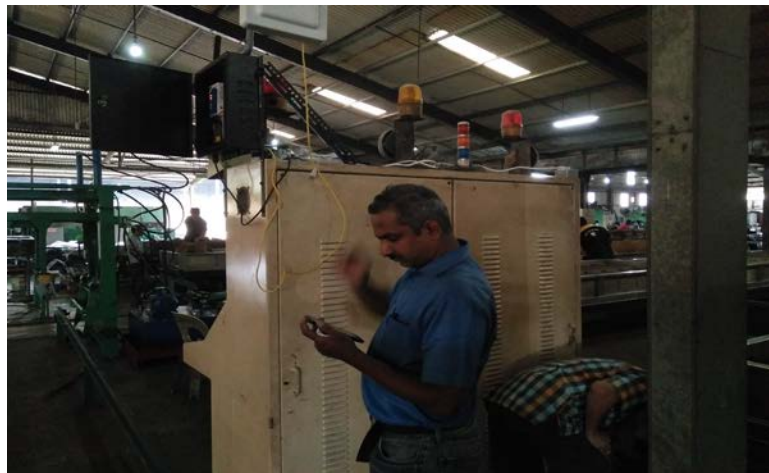
Figure 12. IoT control panel and router box
