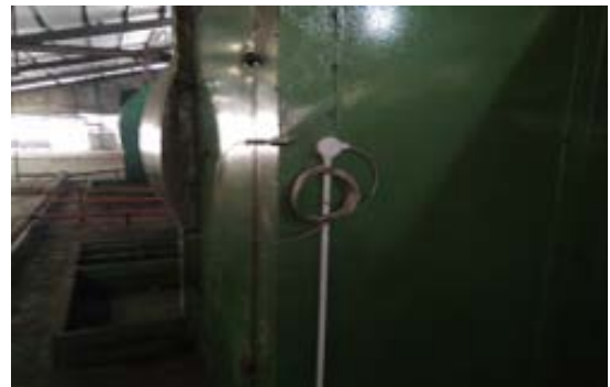
Figure 9b. Dryer fan (outgoing)
